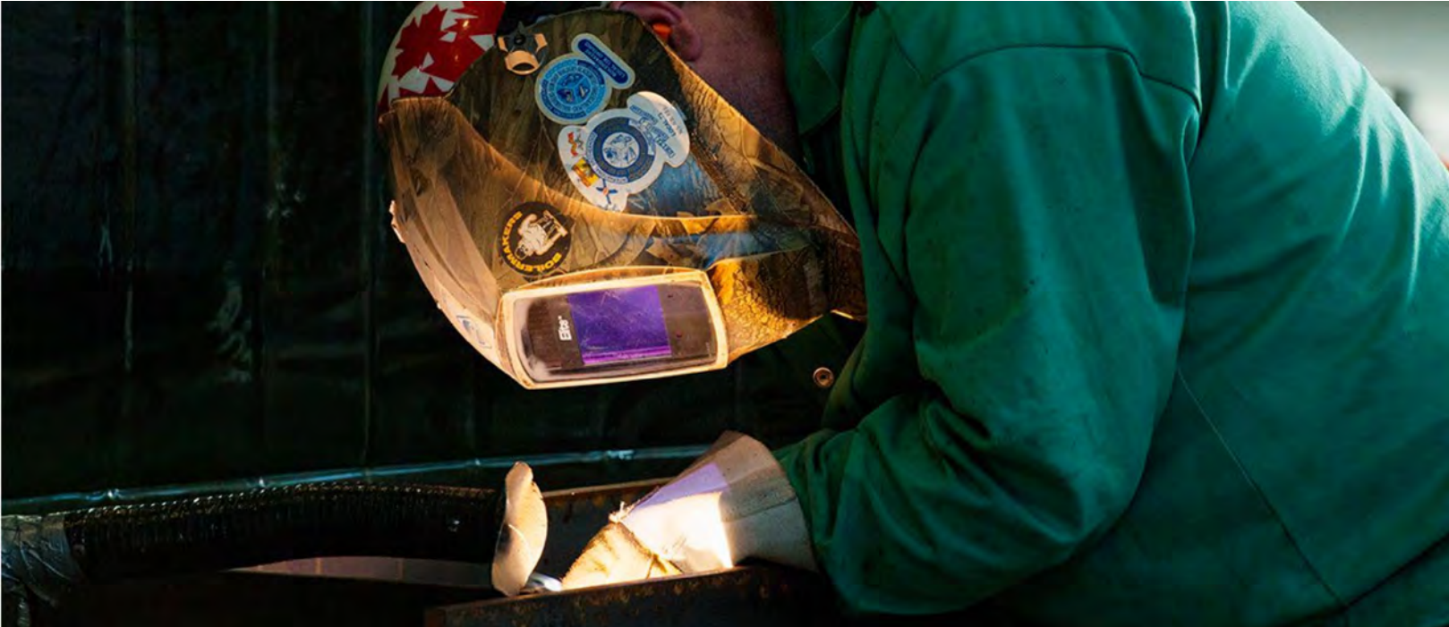
From rebuilding reactor chambers to installations of storage vessels, conduits and cooling systems, Ontario's Boilermakers and other skilled tradespeople, within the nuclear supply chain, played a significant role in the Darlington Unit 2 Refurbishment. Photos courtesy of Ontario Power Generation.
