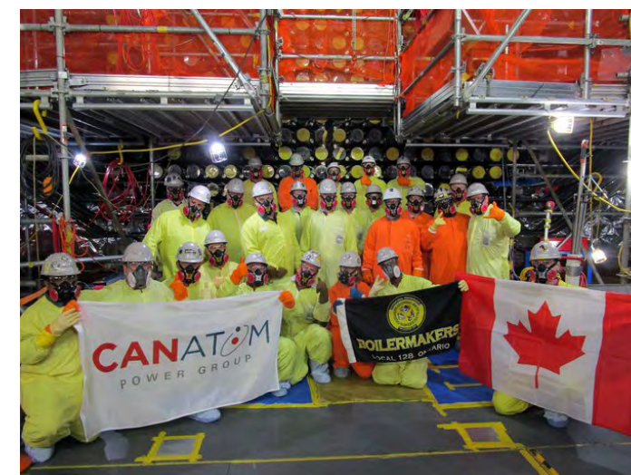
Workers celebrate the successful installation of Darlington Unit 2's 960 feeder tubes in October 2019. This was followed in December by the loading of 6,240 new fuel bundles into the reactor core.
