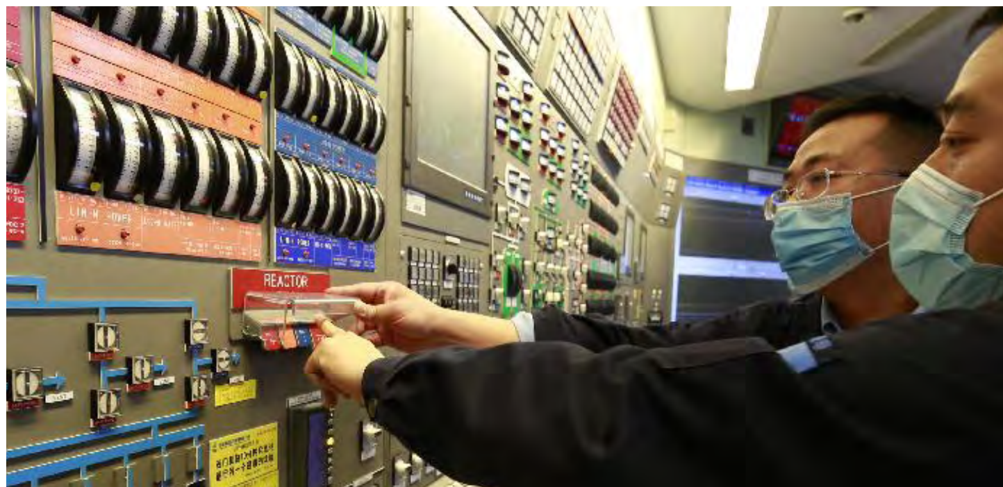
CNNO Third Qinshan Plant staff in the control room where masks were required and access restrictions were in place during the COVID-19 pandemic.
