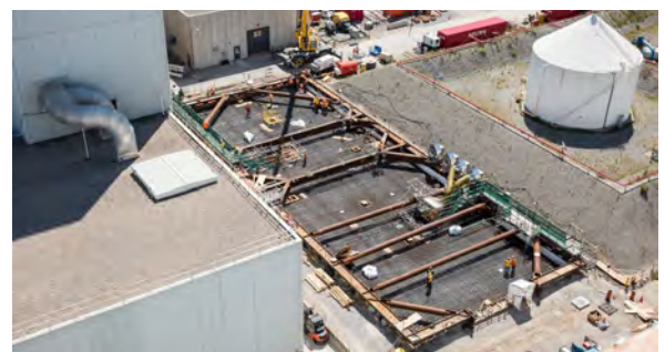
Above: Construction central: Darlington Nuclear has made a multi-million dollar investment in site improvements to support refurbishment and continued operation with 18 new buildings. Top of page: Turbine generator sets will undergo inspection and repair during refurb execution.
