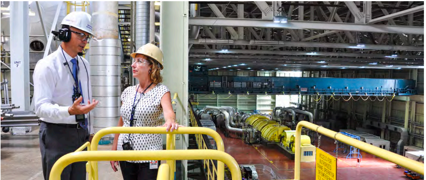
Photo courtesy: Bruce Power
