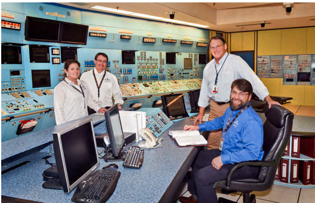
Brett Plummer and the Point Lepreau Nuclear Generating Station team have created a 'teaching' culture to help integrate new staff and re-enforce operationally-focused behaviours in the plant. Above, Plummer (top right) with some members of his team in the PLNGS training simulator. (l-r): Leah Belding, Shift Supervisor-in-Training, Gerry Fairweather, Shift Supervisor and John McNiven, Licenced Control Room Operator.
