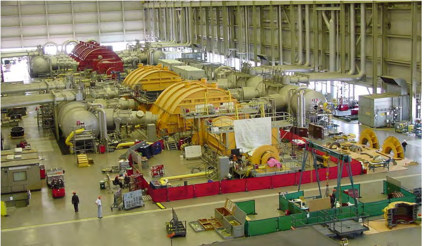
Darlington Unit 2 (above) is in execution phase. Several of the plant's 58 systems have already been restarted and reassembly has begun.
